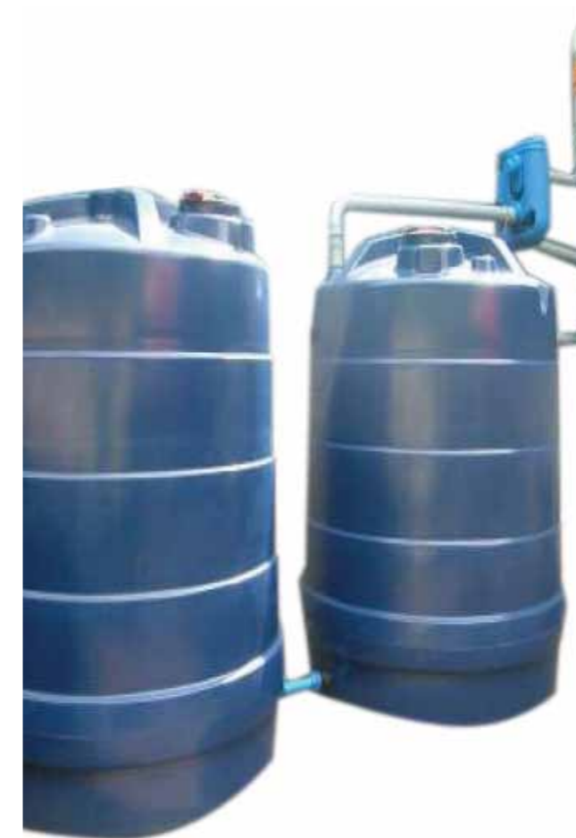
Figure 4 → Examples of above ground storage tanks
