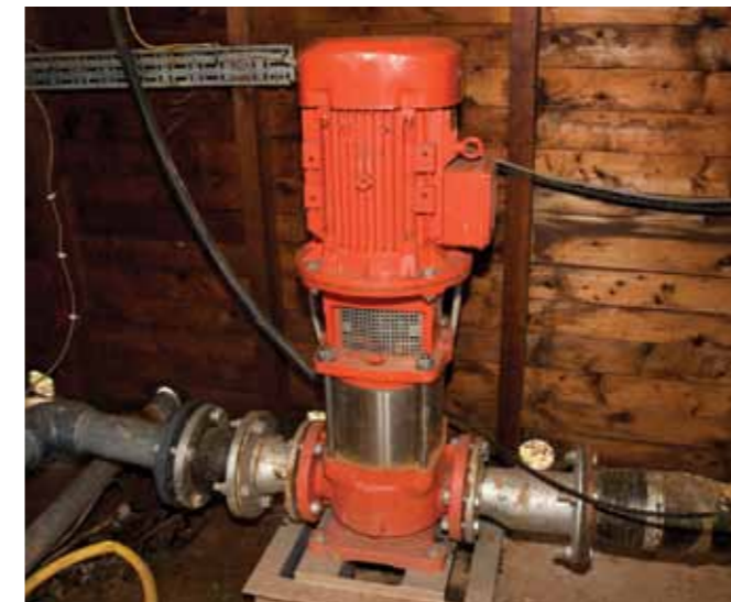
Pumps are needed to ensure the right pressure for the use of water
