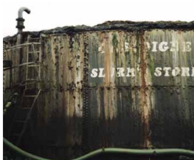
You can reduce the size of the slurry store that you need if you divert clean roofwater away from the store
