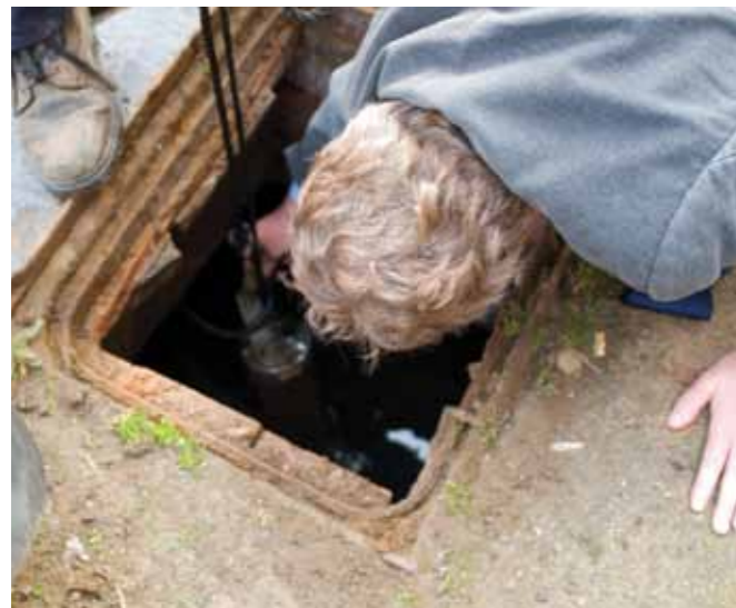
In underground storage tanks ensure you can access the pump for maintenance
