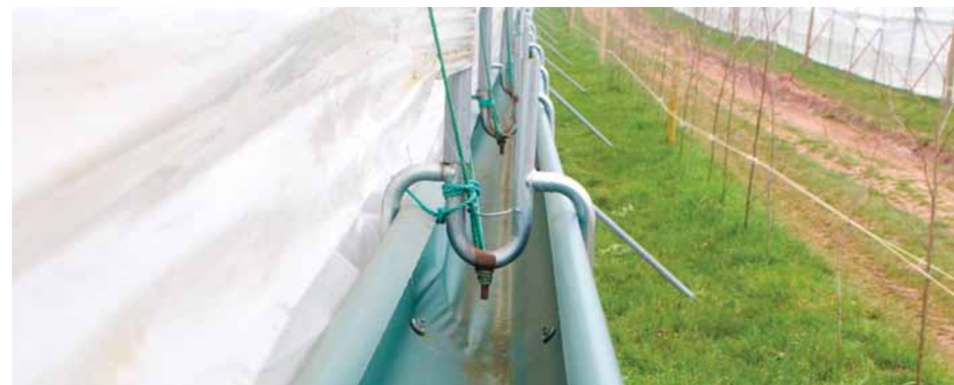
Good guttering is vital to capture rainwater
